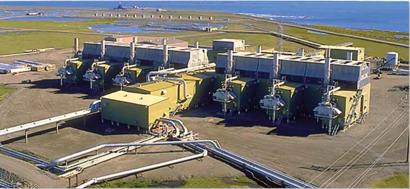
The central compressor plant at Prudhoe Bay, where high volumes of safe and reliable CO 2 injection has been practiced for three decades.
